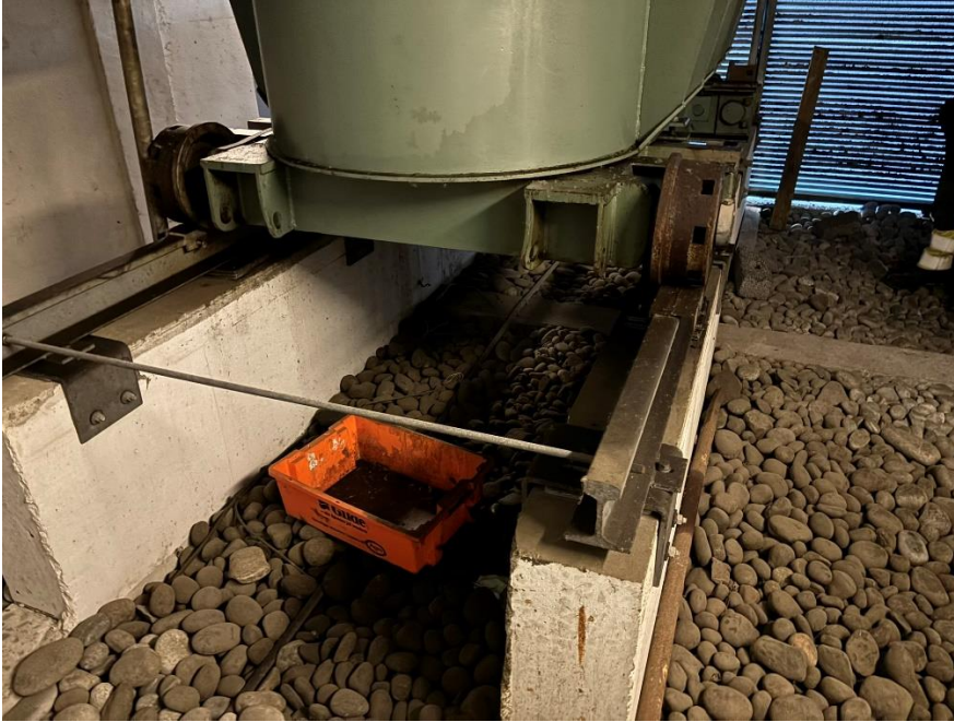
Figur 2: Steinfilter i T1.
